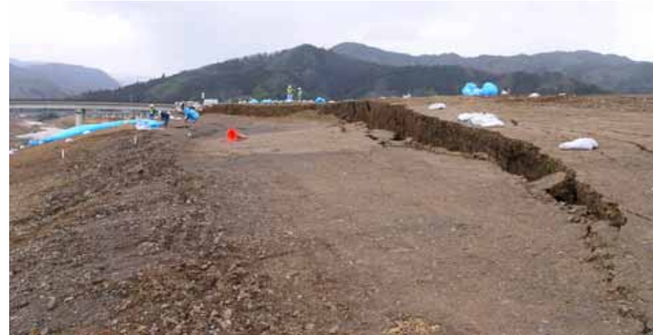
堤防天端の亀裂
