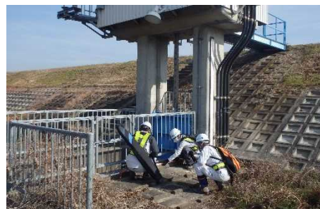
▲樋門周辺護岸の沈下を点検
