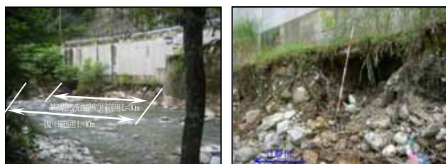
軽量盛土前面の洗掘範囲
