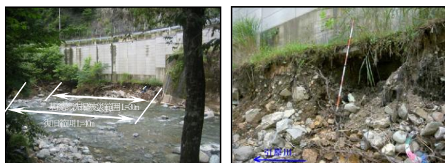
軽量盛土前面の洗掘範囲
