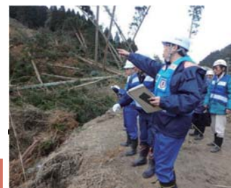
Local Government Support Activities (Technical support by TEC-FORCE, Miyazu City, Kyoto Prefecture)
