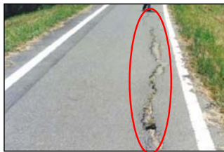
堤防天端の亀裂
