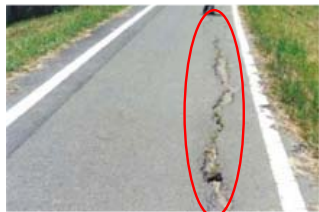
堤防天端の亀裂
