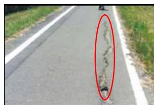
堤防天端の亀裂
